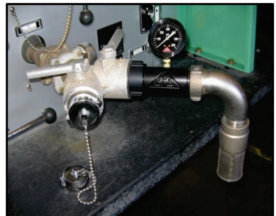
Figure 10. Pressure valve attached to the footvalve.
